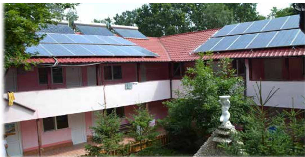
Fig. no. 4 - Photovoltaic panels
