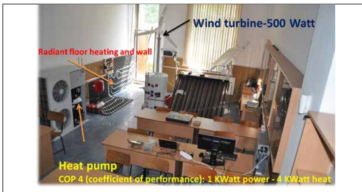
Fig. no. 2 - Renewable energy laboratory [1]
