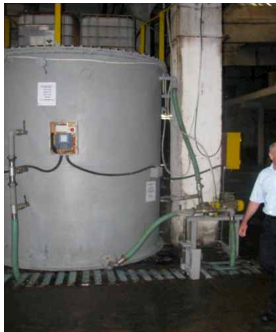
Figure 1. Industrial installation (12-14m 3 ) of residual float exhaustion from leather tanning
